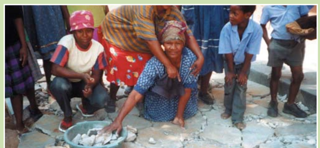
Loxey community salvaging and reusing concrete from Loxey Primary School renovations, South Africa.
